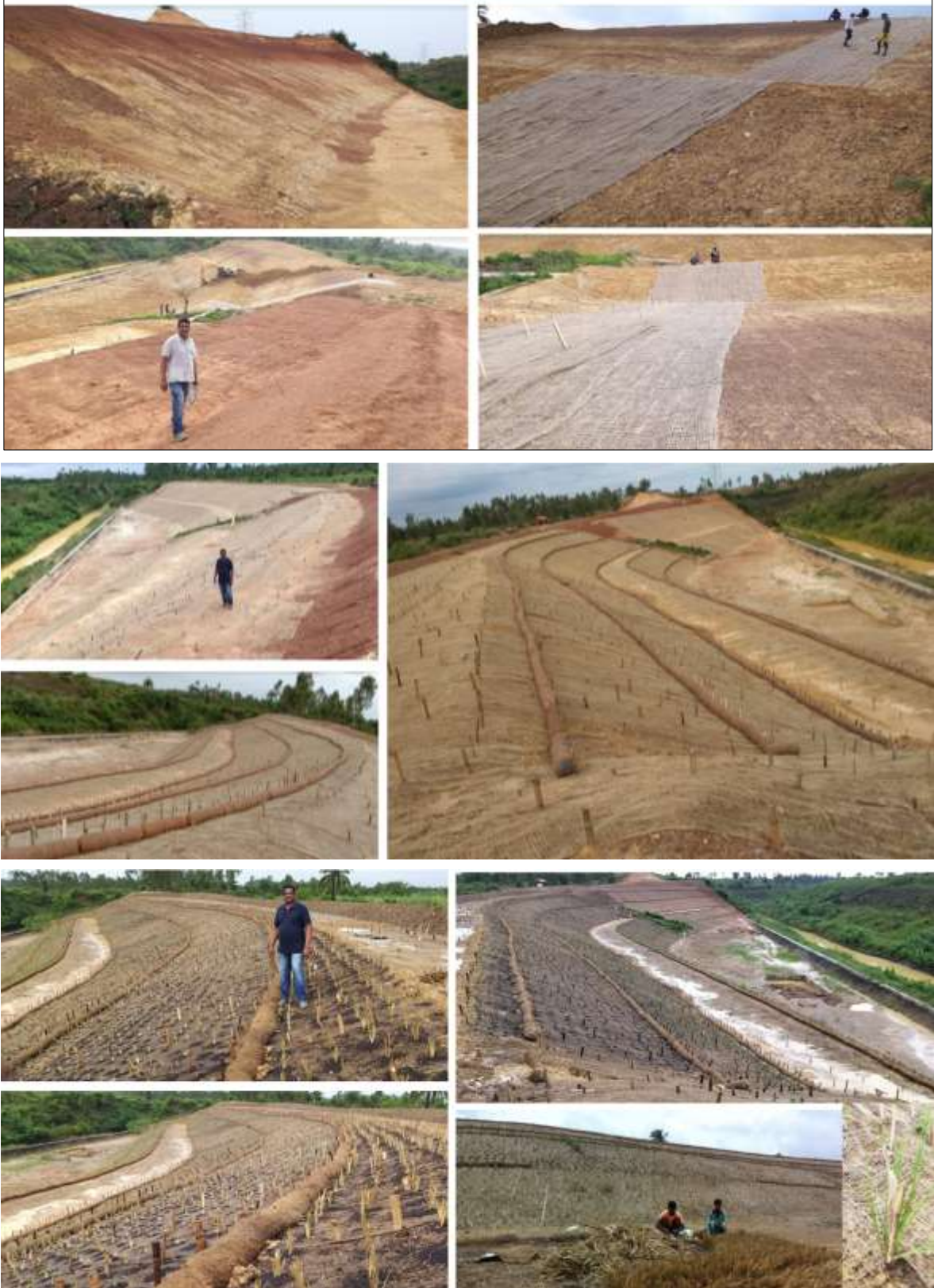
Slope stabilization using bioengineering solutions Project consultant to IRRIGATION & WATERWAYS DEPARTMENT ( I&WD), Govt. of West Bengal
